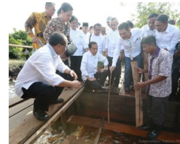
President Joko Widodo inspects the canal blockages constructed by local communities in Sungai Tohor village, Tebing Tinggi Subdistrict. The canal blockages are able to prevent peatlands from draining process, thereby reducing the risk of fires. (Meranti, Riau, 27 November 2014)
